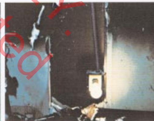
7 This photo shows same receptacle as photo #5, but the wall board was removed to show wiring and box intact. See Diagram II.
