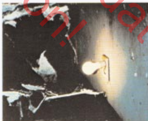
5 This receptacle is located in room 206 and is operative after flashover. Room temperatures during flashover shown in Graph B. See Diagram II.
