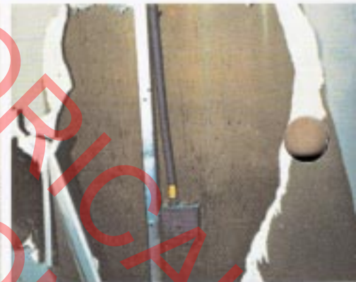
2 This is the reverse side of photo #1 showing the reverse side of the wall and tubing intact and undamaged. See Diagram II.
