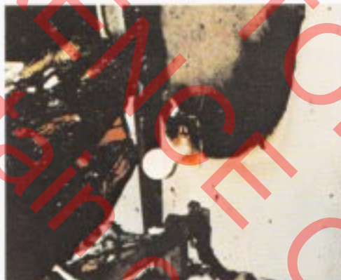
1 This wall receptacle in the apartment master bedroom shows the extent of fire damage to bed frame, wall and outlet plate, while circuit operation is demonstrated by light. Recorded room temperatures are shown in Graph A. See Diagram II.
