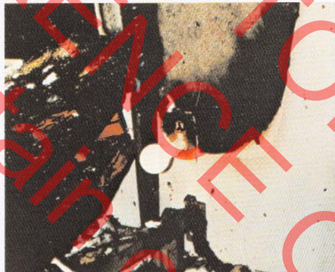
1 This wall receptacle in the apartment master bedroom shows the extent of fire damage to bed frame, wall and outlet plate, while circuit operation is demonstrated by light. Recorded room temperatures are shown in Graph A. See Diagram II.
