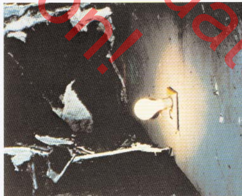
6 This receptacle is located in room 206 and is operative after flashover. Room temperatures during flashover shown in Graph B. See Diagram II.
