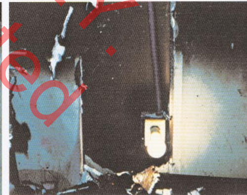
7 This photo shows same receptacle as photo 6, but the wall board was removed to show wiring and box intact. See Diagram II.
