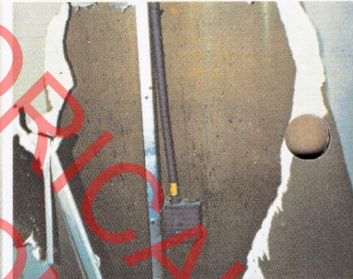
2 This is the reverse side of photo #1 showing circuit box and tubing intact and undamaged. See Diagram II.
