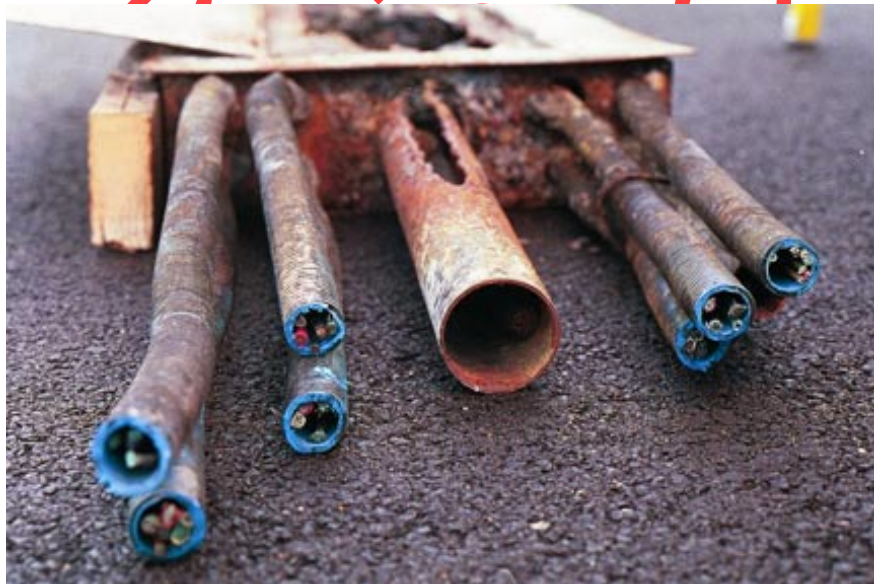
Figure 14: Collateral damage to metal and ENT raceways. San Jose, California
