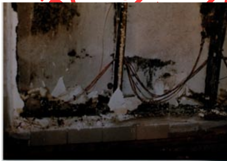
Figure 42: Same specimen after 30 minute fire exposure
