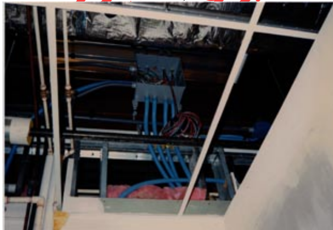
Figure 11: Distribution box in Marriott Hotel project Cleveland, Ohio
