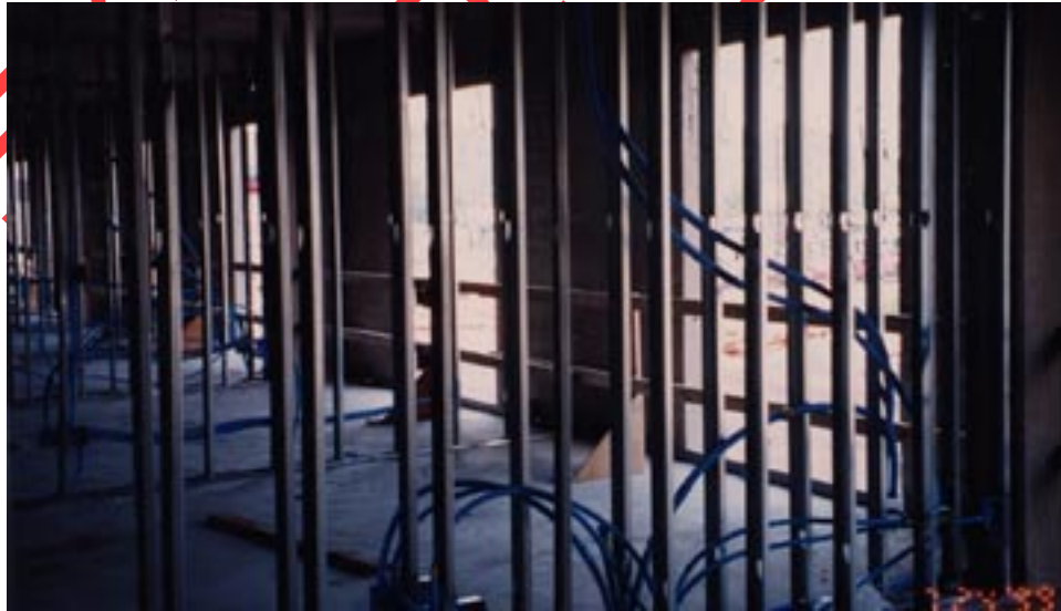
Figure 55: ENT used in steel stud walls prior to installation of gypsum wallboard
