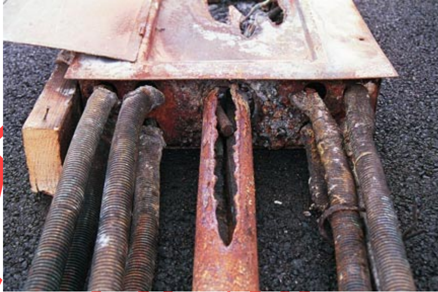
Figure 17: Condition of conductors after fire in ENT and Rigid Metal Conduit (RMC) San Jose, California
