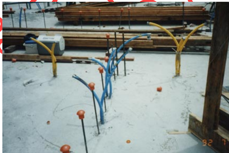
performance run from non- Figure 19: ENT stubbed out from concrete slab under construction
