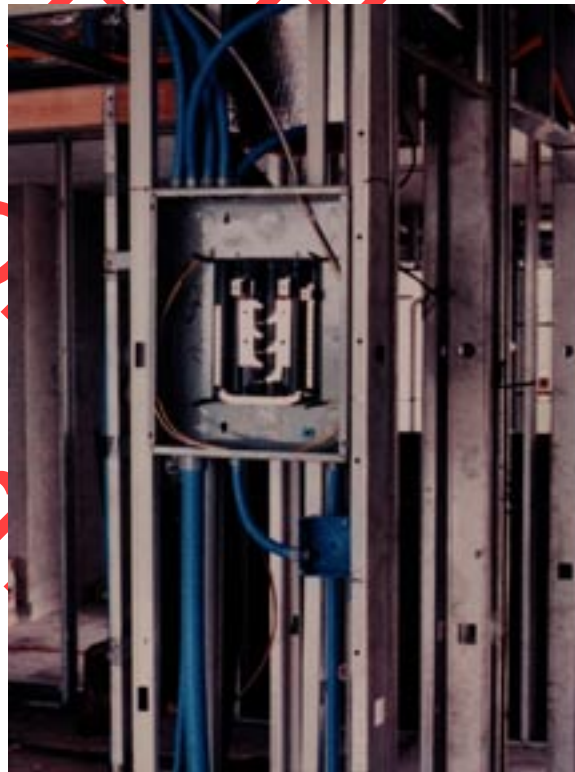
Figure 48: ENT installed in sub-panel location of highrise apartment complex, Patterson, New Jersey
