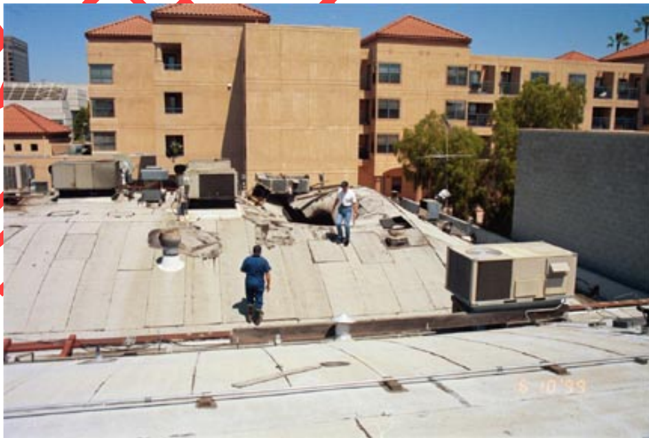
Figure 12: Post-fire view of restaurant roof: fire plume penetrated roof at center of photo. San Jose, California
