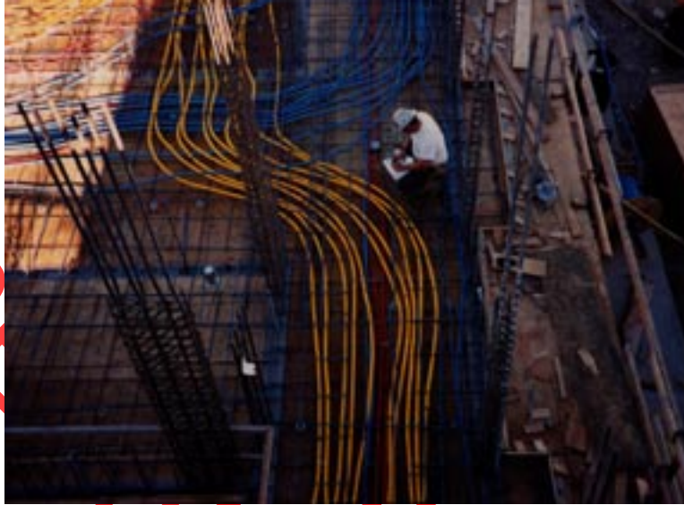
Figure 51: ENT installed in highrise hotel-Four Seasons, Southern California
