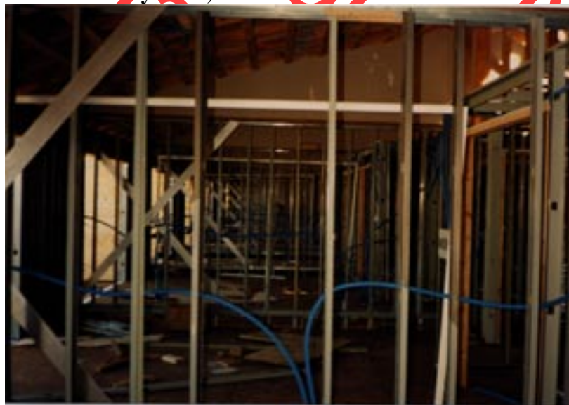
Figure 8: ENT use in type V construction Penta Hotel, Orlando, Florida
