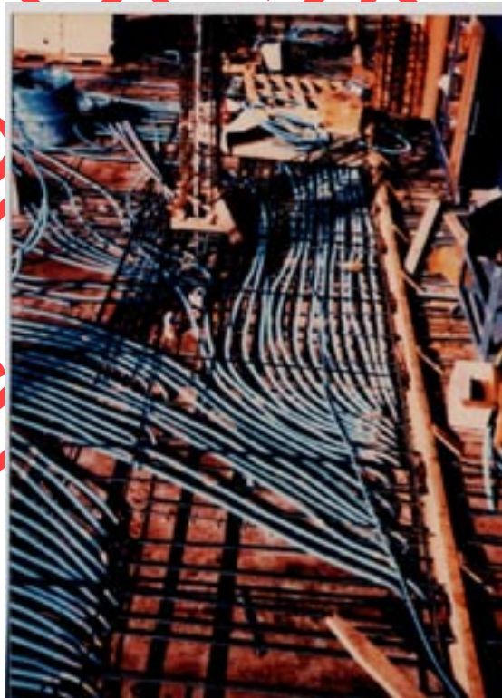
Figure 50: ENT being installed prior to concrete pour in highrise structure, Southern California
