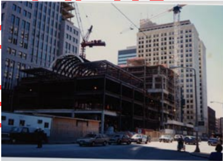
Figure 10: Marriott Hotel project using ENT products Cleveland, Ohio
