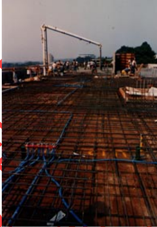
Figure 52: Pouring concrete with ENT installed in highrise apartment complex, Patterson, New Jersey
