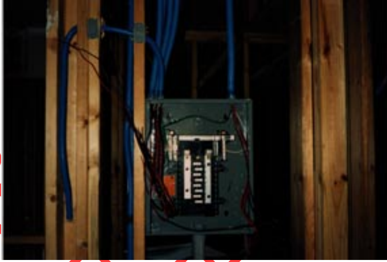
Figure 32: Distribution panel with ENT
