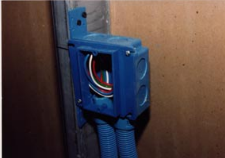
Figure 34: Wired PVC Box and ENT installed in ASTM E-119 wall test assembly
