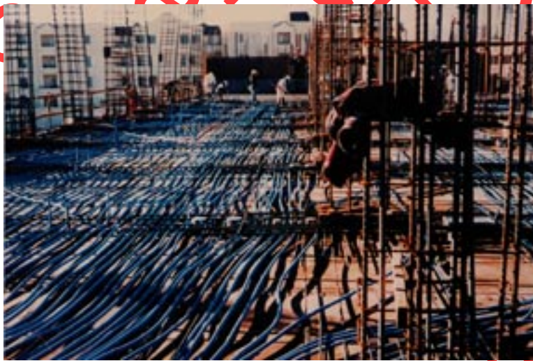
Figure 53: ENT installed on top floor of highrise structure, Southern California
