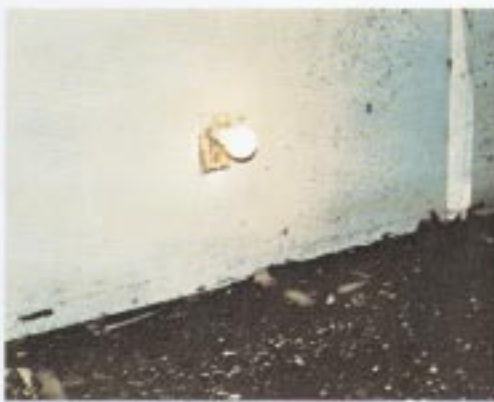
9 Outlet box in Blue Ballroom still functioning after final room burn (flashover). Temperatures are recorded in Graph C. See Diagram I.
