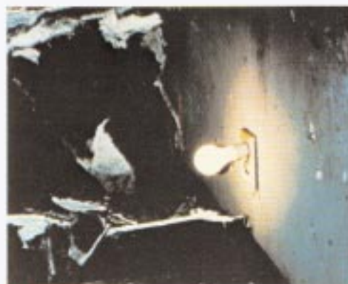
⑥ This receptacle is located in room 206 and is operative after flashover. Room temperatures during flashover shown in Graph B. See Diagram II.
