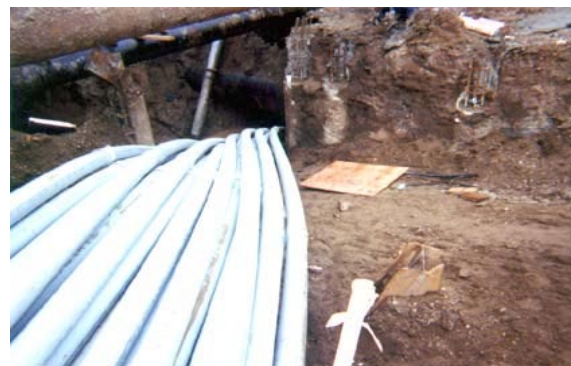
Above Right: Twenty-Six 4" Bore-Gard conduits and four 4" Boreable Multi-Gard ducts, each 200 ft. long, are being pulled through a 200 ft. long bore.
