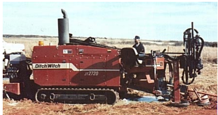
At Left: In the foreground is the reamer attached to the drill string. Barely visible from 1,000 feet on the horizon is the drilling machine. Above Right: A close-up look at the powerful Ditch Witch ® JT2720 that quickly and easily pulled in the 1,000 ft. string of Bore-Gard.
